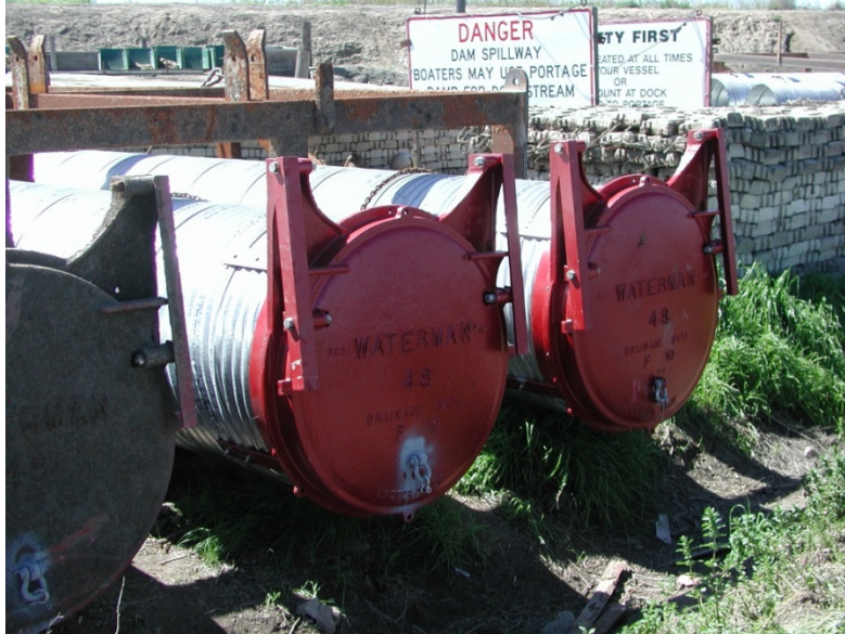
Figure 1-2 The Culverts with Flap Gates at the Old River Tracy Barrier
