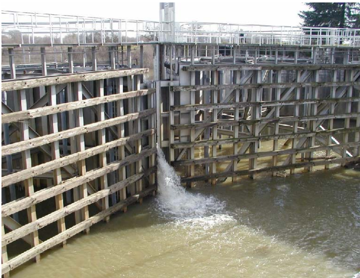
Figure 2.3: Water leaking through the closed boat lock.
